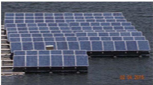
Fig. 3: 30.6 KW PLANT AT WALVAN DAM
